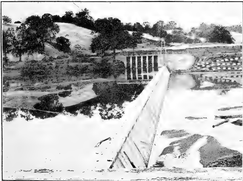
FIG. 2.—SPILLWAY OF DIVERSION DAM NEAR WOODLAND, CALIF. Showing holes along center line of crest to receive flashboard pins.
